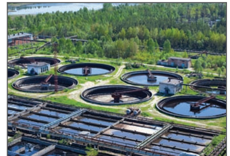
Water, wastewater treatment
